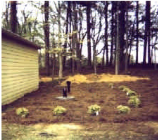
Figure 4: Exterior picture of the Life Pod unit buried underground and surrounded by landscaping.
